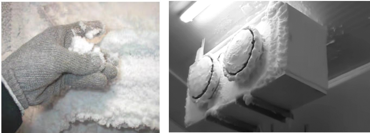
Figure I.17: Unfavorable frost forming due to the presence of supersaturated air or/and a high coil temperature difference.
