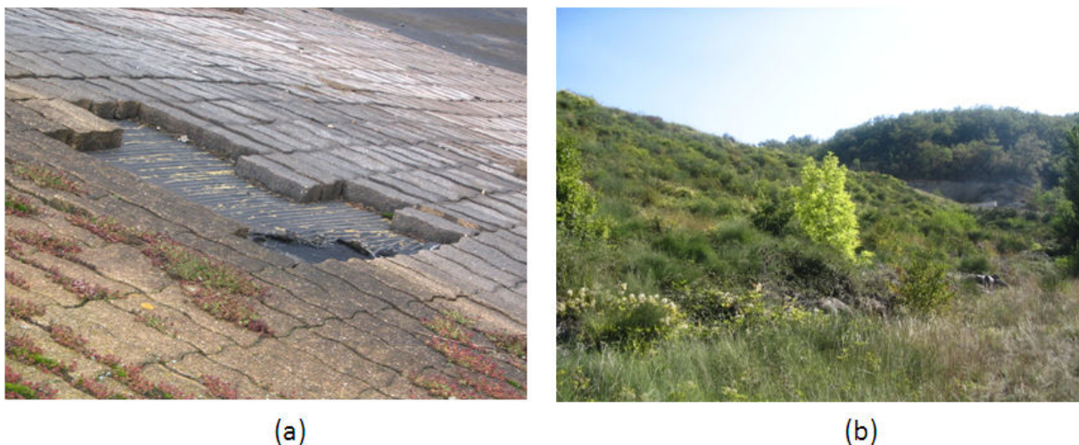
Figure 6.1: Examples of deterioration phenomena - Photos Irstea
