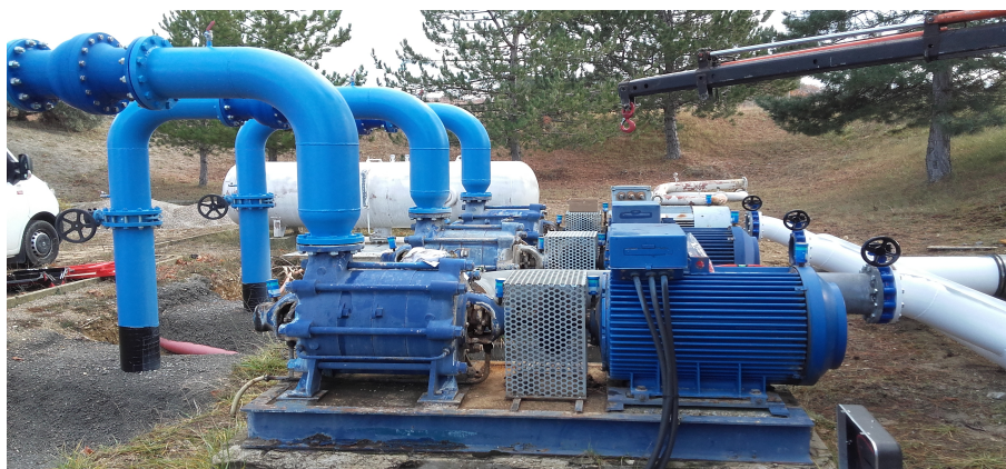
Figure 1.2 – Station de pompage
